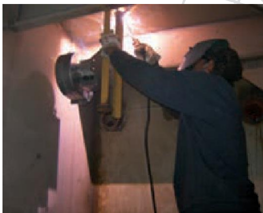
Welding produces poisonous fumes. Here it is not removed.
