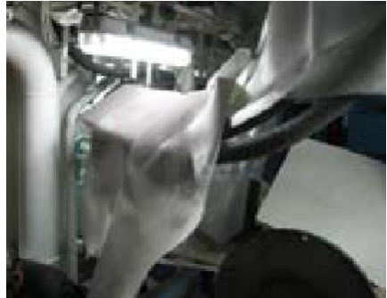
Protection against sparks at hot work.
