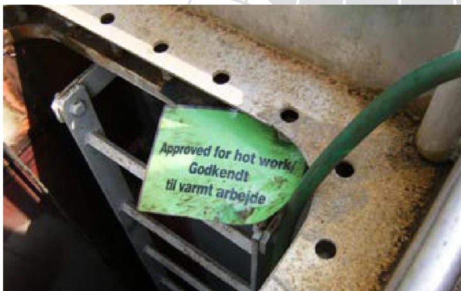
Seal that shows the tank is ready for hot work.
